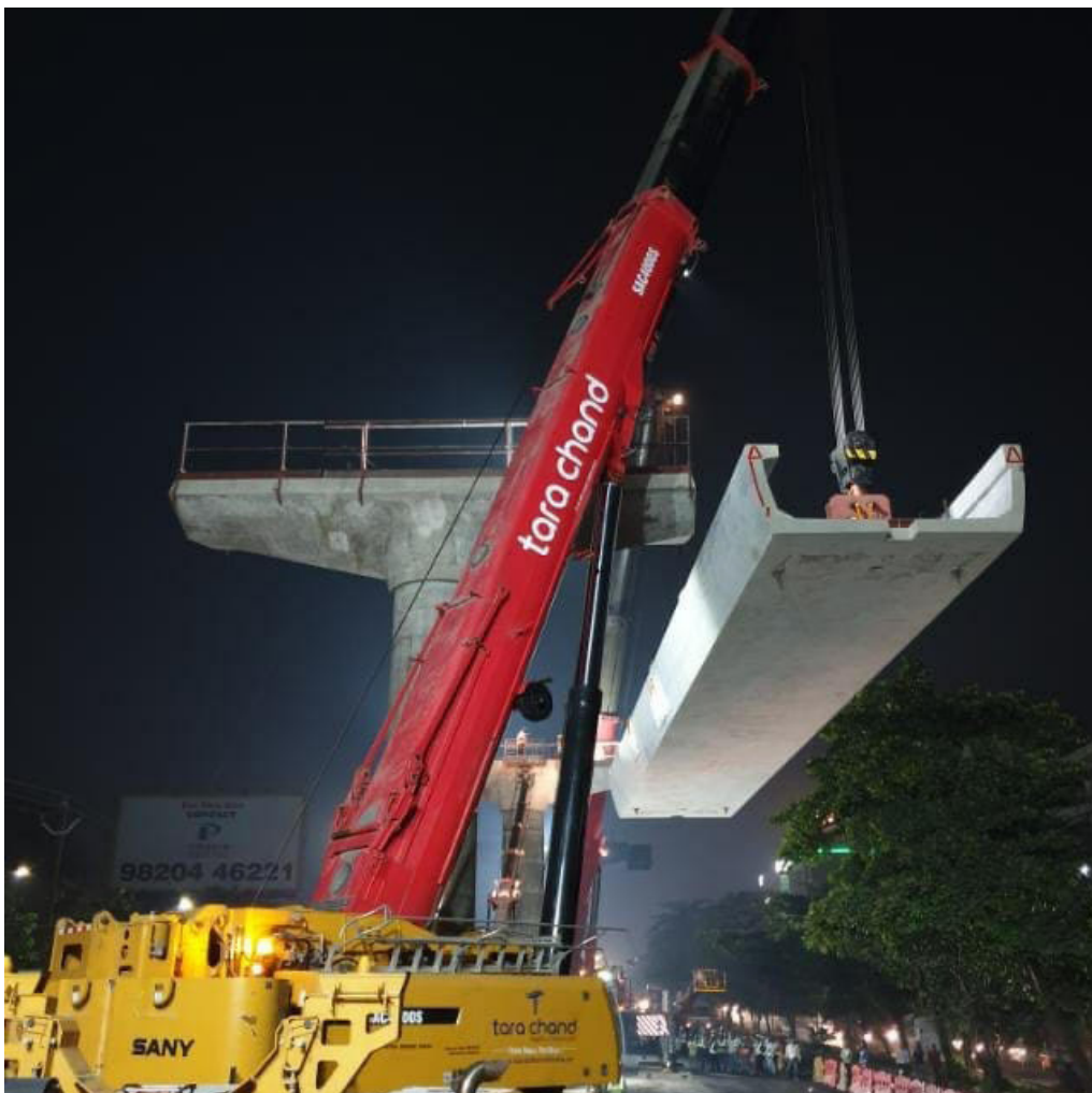
Our Proficient team carrying our Viaduct U Girder Erection work at Mumbai Metro
