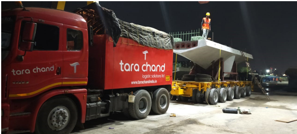
Casted Pier Cap ready to move to Erection Site under our End-to-End Infra Solutions service package
