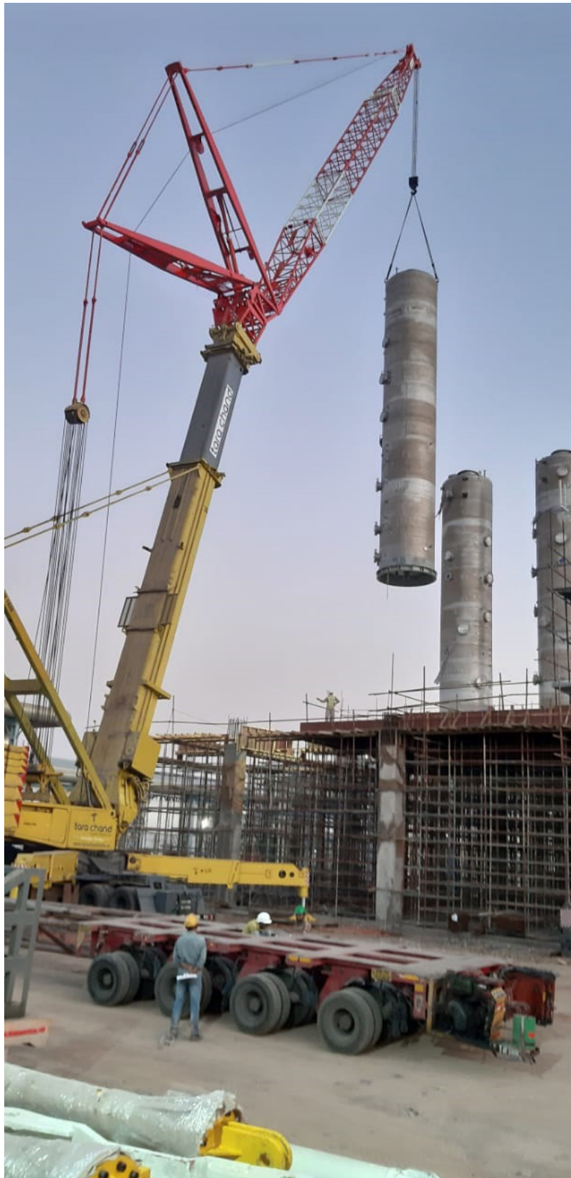
Our 800MT Liebherr LTM1800 Crane executing critical lift at a Cement Plant in Gujarat
