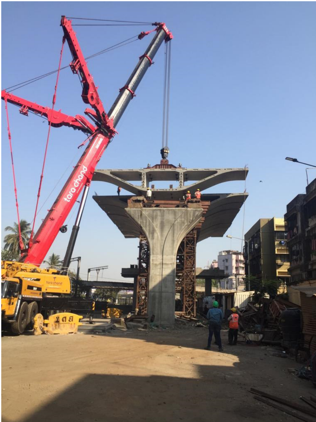
Our professional services and equipment engaged in critical flyover erection works in Mumbai
