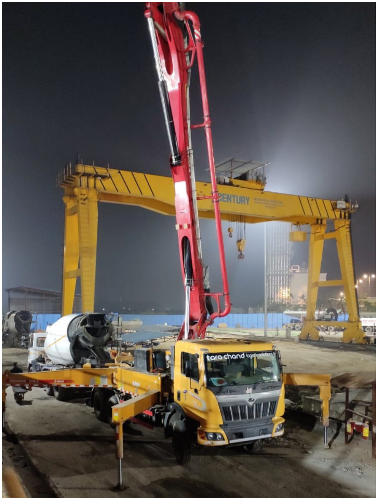
Our Concrete Boom Placer executing critical casting of Viaduct U-Girder at Mumbai Metro
