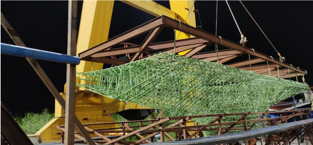
Our Team readying a Viaduct Pier Cap for casting at Mumbai Metro Project
