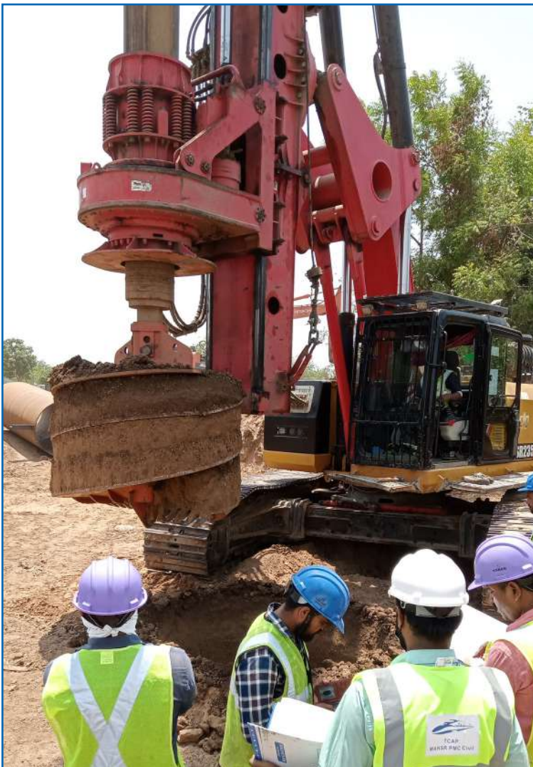
SANY SR235 (235 KNm) Piling Rigs and Engineering Team working at MAHSR Bullet Train Project.
