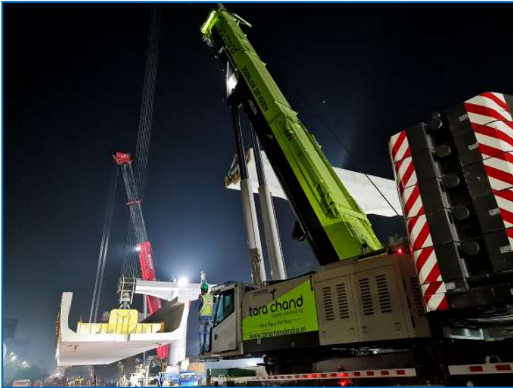
Our Equipment and Teams in action for Metro Rail Construction projects in Mumbai
